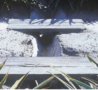
Surface drainage structures such as v-drains can help divert run-off into stable waterways
